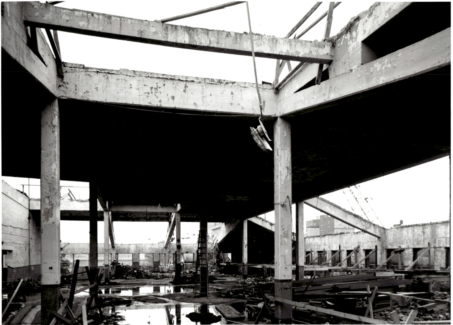
ACADEMIC CENTER UNIVERSITY OF BALTIMORE ROY KIRBY & SONS, INC., CONTRACTOR FISHER, NES, CAMPBELL & PARTNERS, ARCHITECTS REMOVAL OF EXISTING ROOF NOVEMBER 4, 1970
