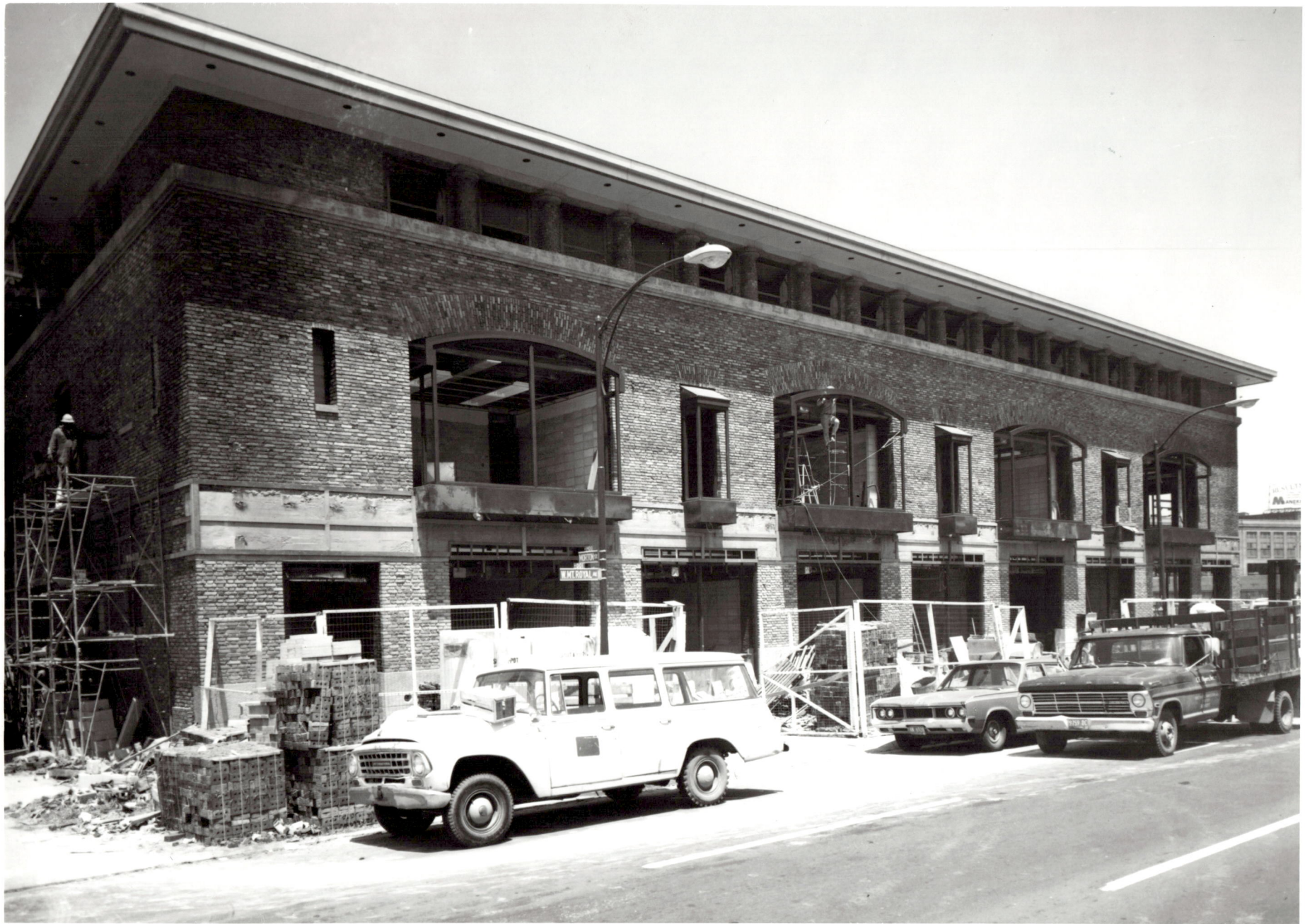
ACADEMIC CENTER UNIVERSITY OF BALTIMORE ROY KIRBY & SONS, INC., CONTRACTOR FISHER, NES, CAMPBELL & PARTNERS, ARCHITECTS GENERAL VIEW LOOKING NORTHEAST JUNE 1, 1971
