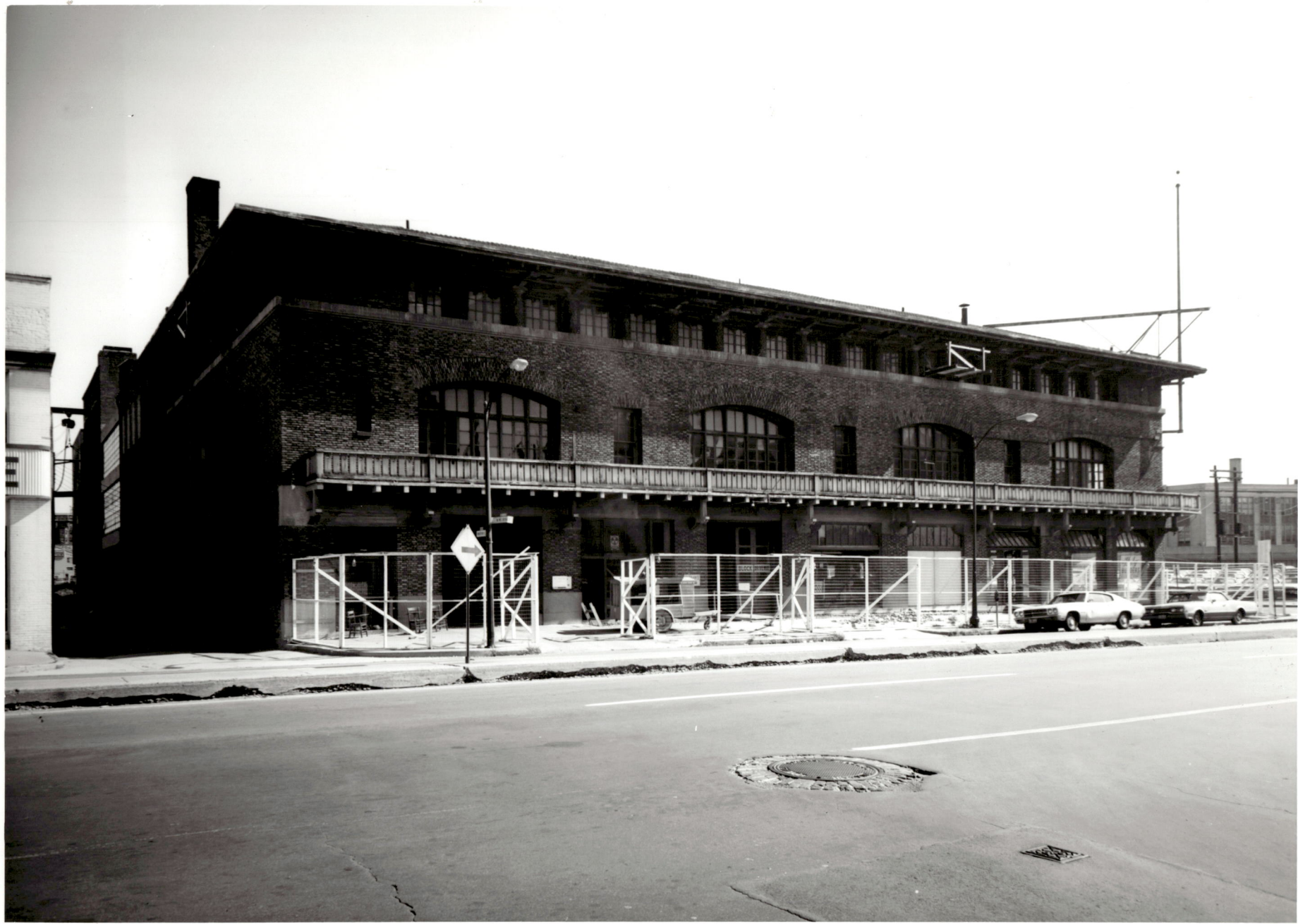
ACADEMIC CENTER UNIVERSITY OF BALTIMORE ROY KIRBY & SONS, INC., CONTRACTOR FISHER, NES, CAMPBELL & PARTNERS, ARCHITECTS GENERAL VIEW LOOKING NORTHEAST AUGUST 4, 1970
