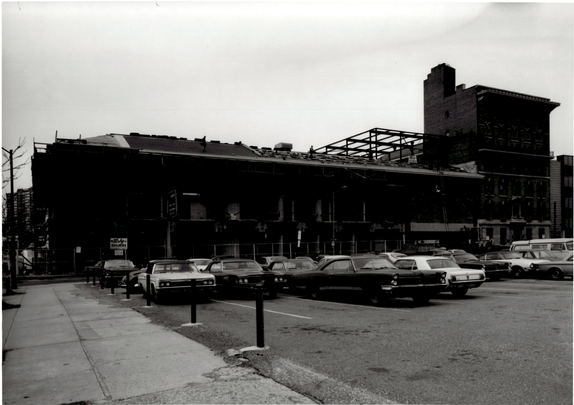
ACADEMIC CENTER UNIVERSITY OF BALTIMORE ROY KIRBY & SONS, INC., CONTRACTOR FISHER, NES, CAMPBELL & PARTNERS, ARCHITECTS LOOKING NORTHWEST FROM MT. ROYAL AVENUE AT SLATING ON ROOF APRIL 1, 1971
