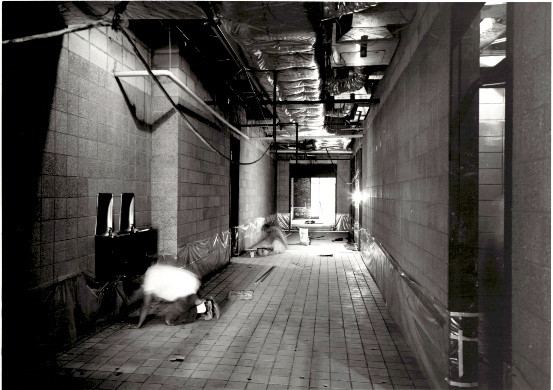
ACADEMIC CENTER UNIVERSITY OF BALTIMORE ROY KIRBY & SONS, INC., CONTRACTOR FISHER, NES, CAMPBELL & PARTNERS, ARCHITECTS TERRAZOING HALLWAY JULY 1, 1971
