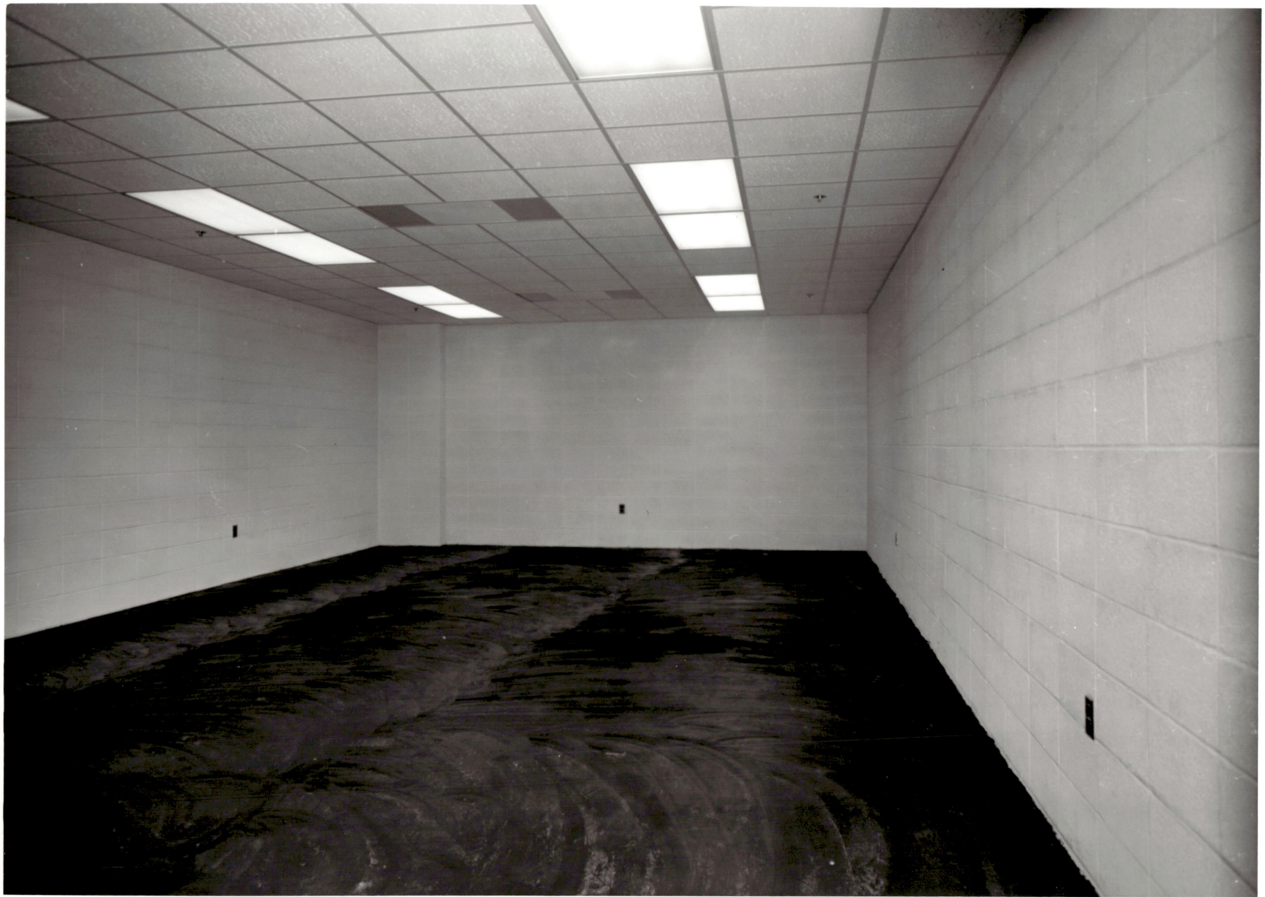
ACADEMIC CENTER UNIVERSITY OF BALTIMORE ROY KIRBY & SONS, INC., CONTRACTOR FISHER, NES, CAMPBELL & PARTNERS, ARCHITECTS CLASSROOM #5 AUGUST 3, 1971
