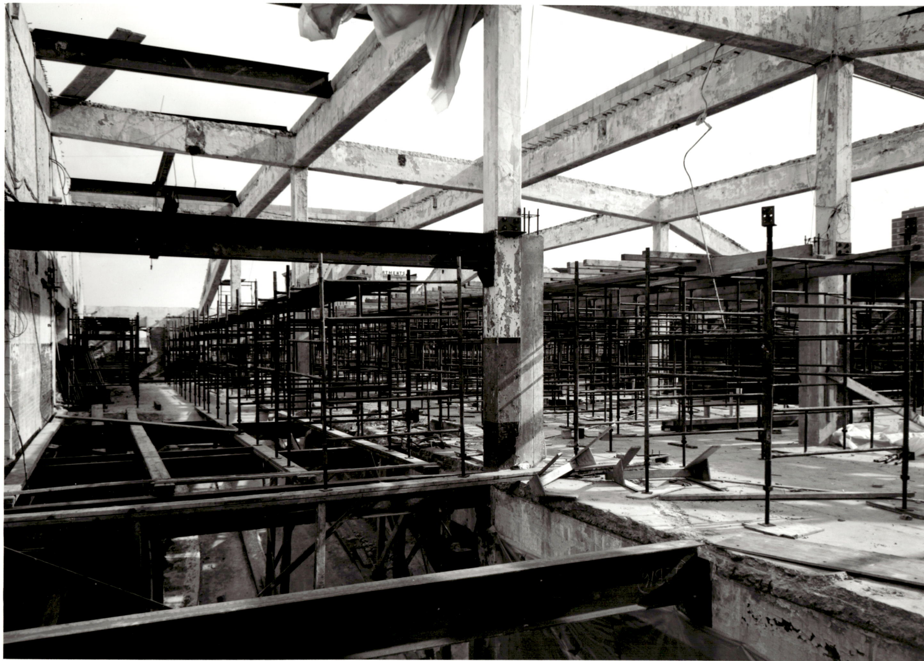
ACADEMIC CENTER UNIVERSITY OF BALTIMORE ROY KIRBY & SONS, INC., CONTRACTOR FISHER, NES, CAMPBELL & PARTNERS, ARCHITECTS SCAFFOLDING - THIRD FLOOR MEZZANINE FEBRUARY 1, 1971
