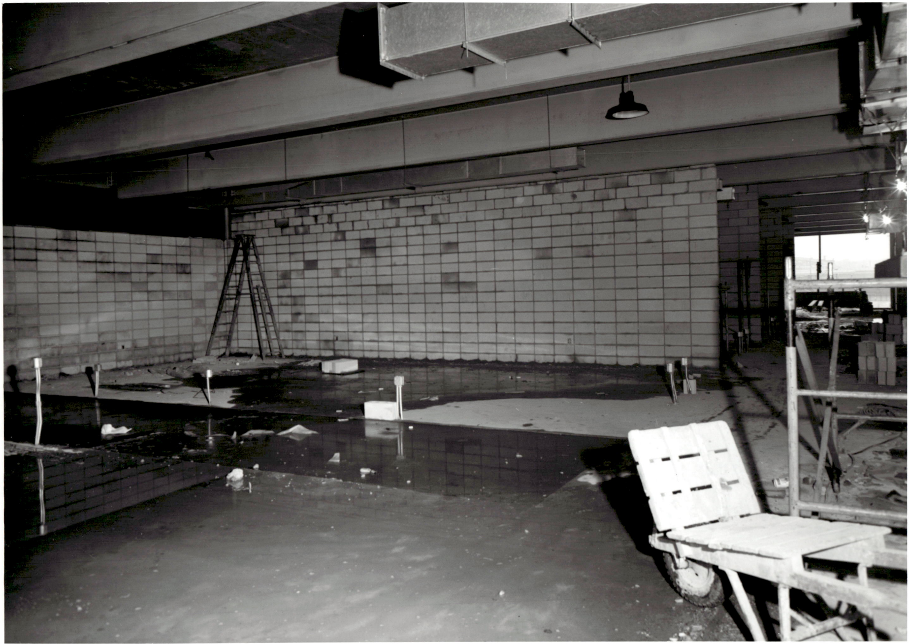
ACADEMIC CENTER UNIVERSITY OF BALTIMORE ROY KIRBY & SONS, INC., CONTRACTOR FISHER, NES, CAMPBELL & PARTNERS, ARCHITECTS BLOCK WALLS GOING UP ON SECOND FLOOR JANUARY 4, 1971
