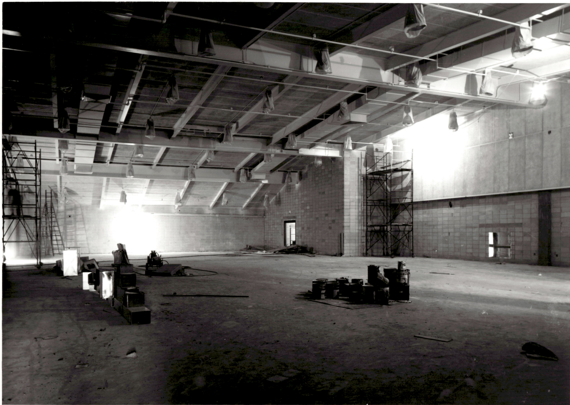
ACADEMIC CENTER UNIVERSITY OF BALTIMORE ROY KIRBY & SONS, INC., CONTRACTOR FISHER, NES, CAMPBELL & PARTNERS, ARCHITECTS PAINTING GYMNASIUM JULY 1, 1971
