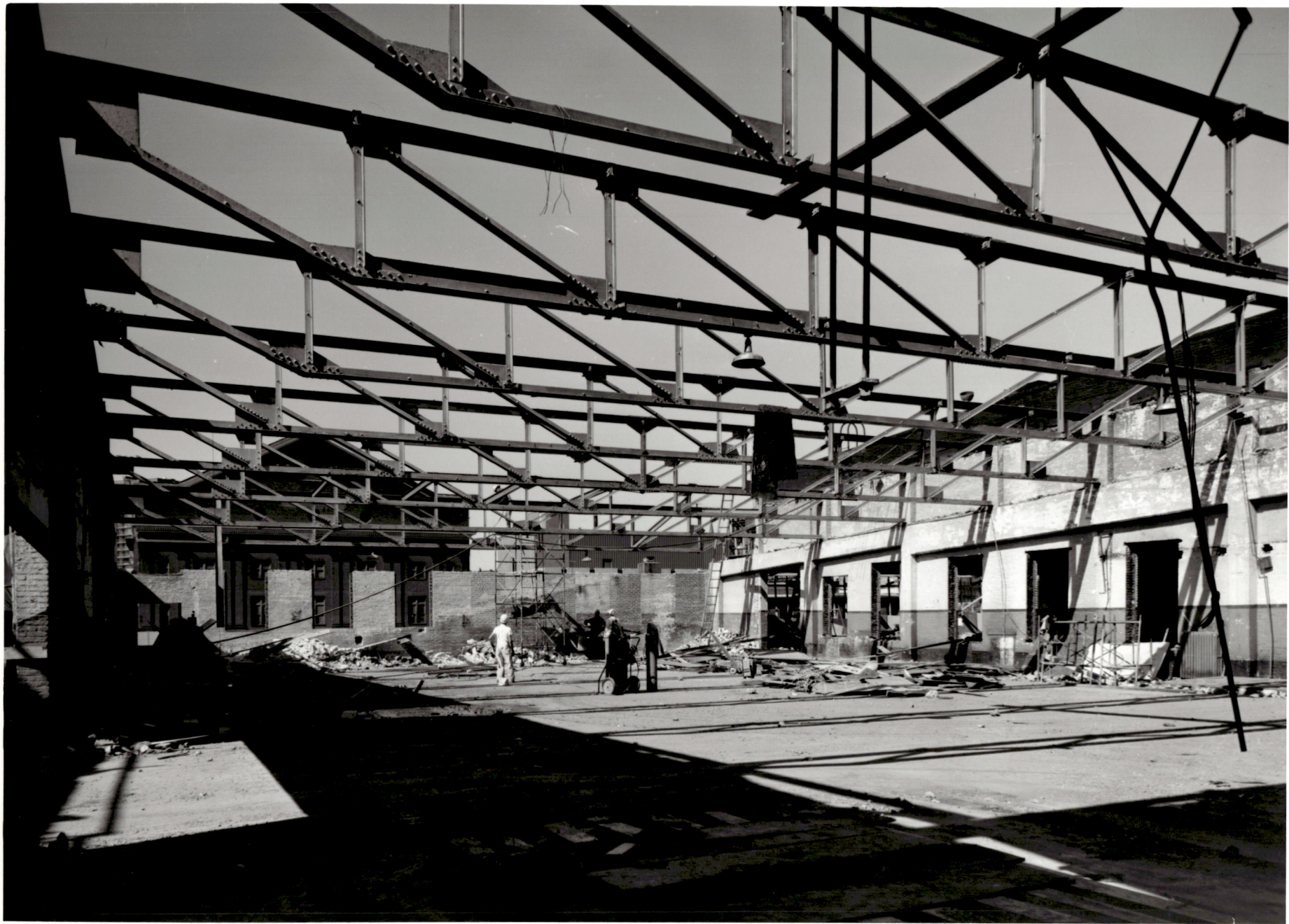
ACADEMIC CENTER UNIVERSITY OF BALTIMORE ROY KIRBY & SONS, INC., CONTRACTOR FISHER, NES, CAMPBELL & PARTNERS, ARCHITECTS REMOVAL OF OLD ROOF OCTOBER 1, 1970
