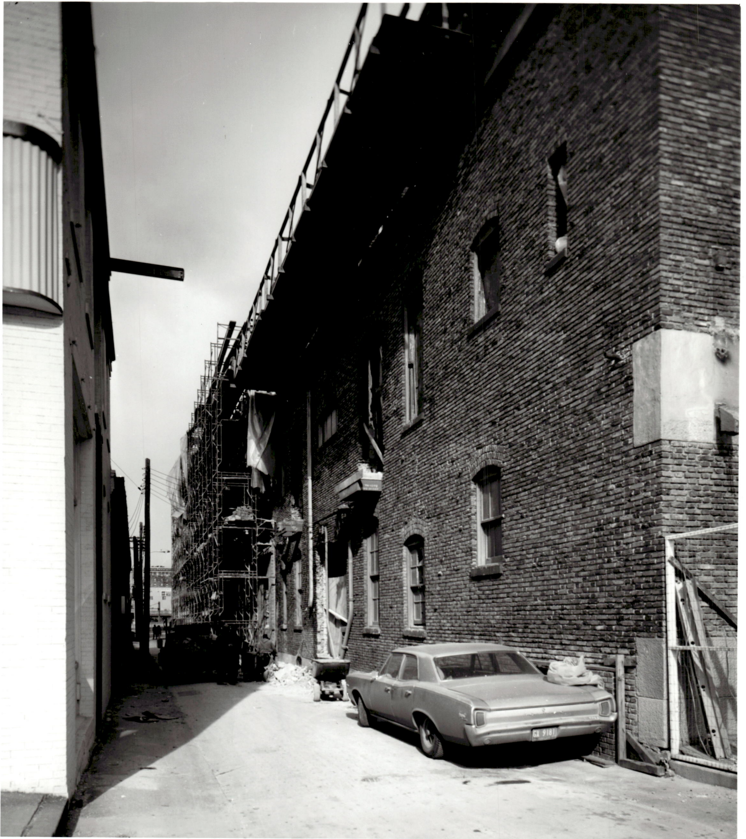
ACADEMIC CENTER UNIVERSITY OF BALTIMORE ROY KIRBY & SONS, INC., CONTRACTOR FISHER, NES, CAMPBELL & PARTNERS, ARCHITECTS SOUTHWEST ALONG CHARLES STREET SHOWING EXTENT OF BRICK WORK FEBRUARY 1, 1971
