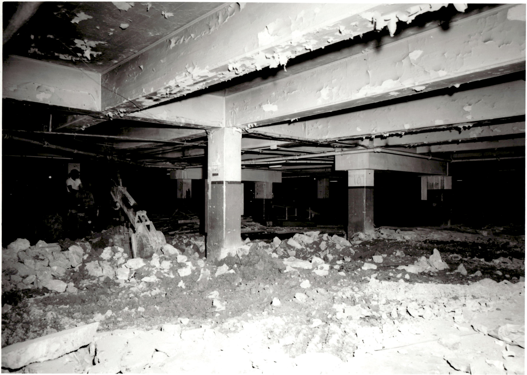
ACADEMIC CENTER UNIVERSITY OF BALTIMORE ROY KIRBY & SONS, INC., CONTRACTOR FISHER, NES, CAMPBELL & PARTNERS, ARCHITECTS BASEMENT LOOKING NORTHWEST AUGUST 4, 1970
