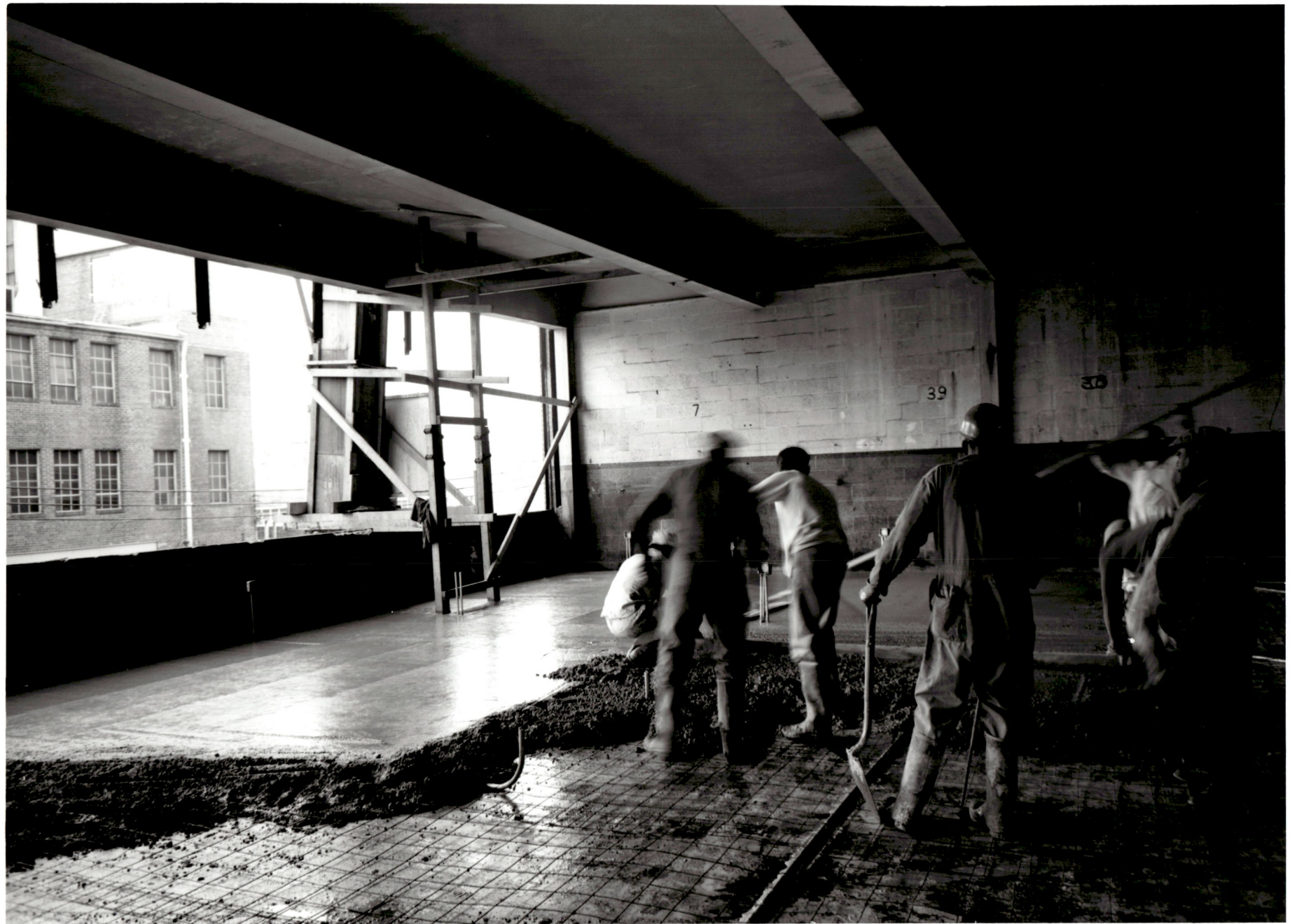
ACADEMIC CENTER UNIVERSITY OF BALTIMORE ROY KIRBY & SONS, INC., CONTRACTOR FISHER, NES, CAMPBELL & PARTNERS, ARCHITECTS POURING NEW DECK SECOND FLOOR NOVEMBER 4, 1970
