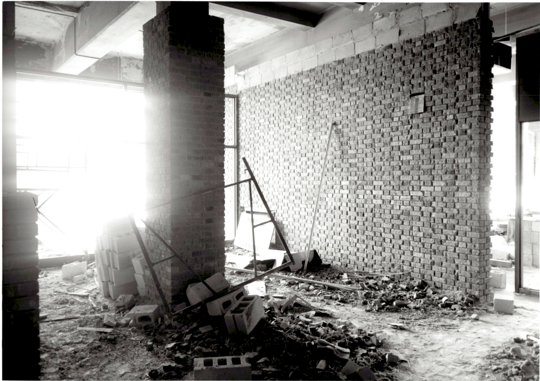
ACADEMIC CENTER UNIVERSITY OF BALTIMORE ROY KIRBY & SONS, INC., CONTRACTOR FISHER, NES, CAMPBELL & PARTNERS, ARCHITECTS LOBBY MARCH 1, 1971
