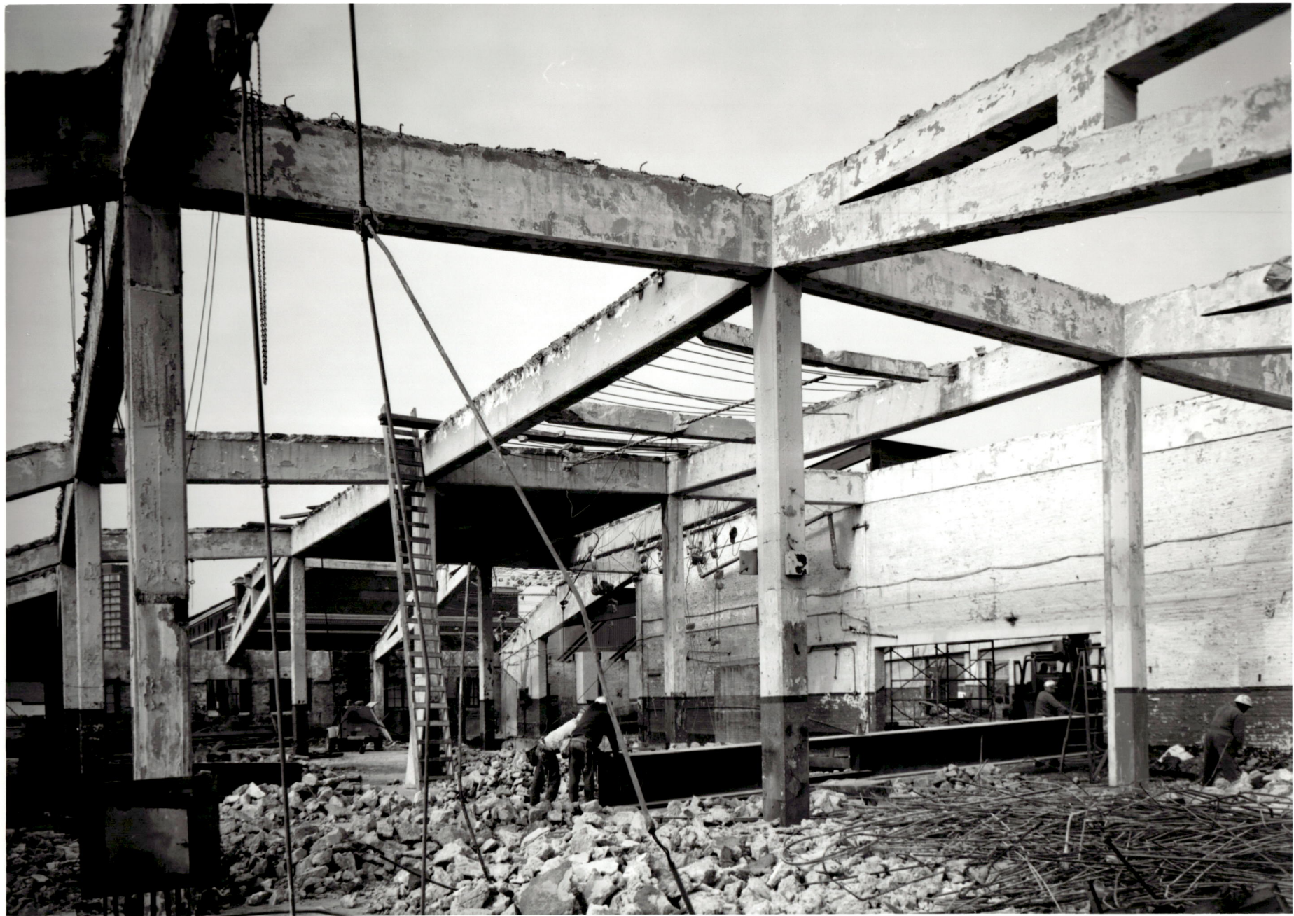
ACADEMIC CENTER UNIVERSITY OF BALTIMORE ROY KIRBY & SONS, INC., CONTRACTOR FISHER, NES, CAMPBELL & PARTNERS, ARCHITECTS REMOVAL OF EXISTING ROOF LOOKING NORTHWEST DECEMBER 1, 1970
