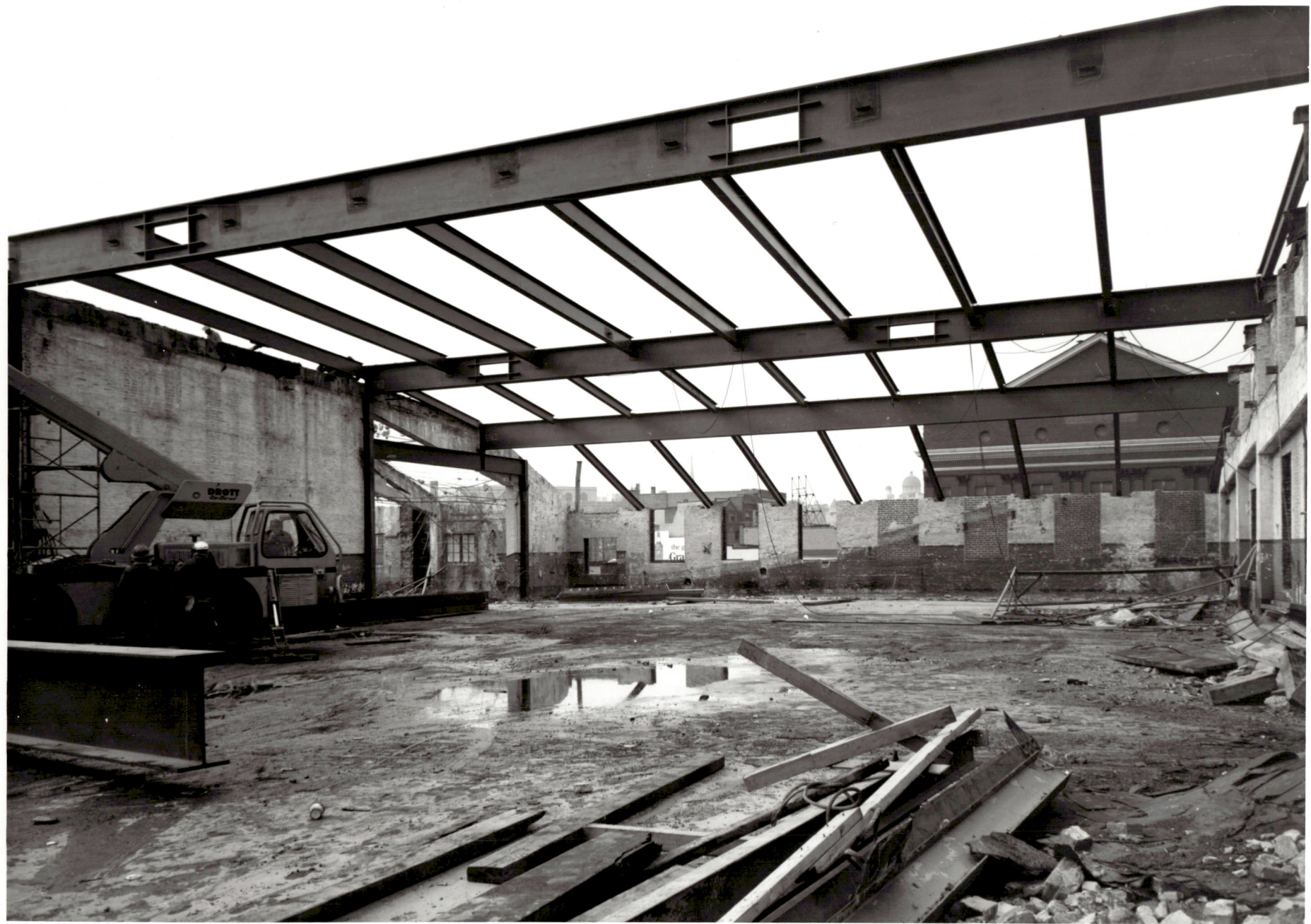
ACADEMIC CENTER UNIVERSITY OF BALTIMORE ROY KIRBY & SONS, INC., CONTRACTOR FISHER, NES, CAMPBELL & PARTNERS, ARCHITECTS GENERAL VIEW LOOKING WEST AT NEWLY INSTALLED STEEL IN ROOF DECEMBER 1, 1970
