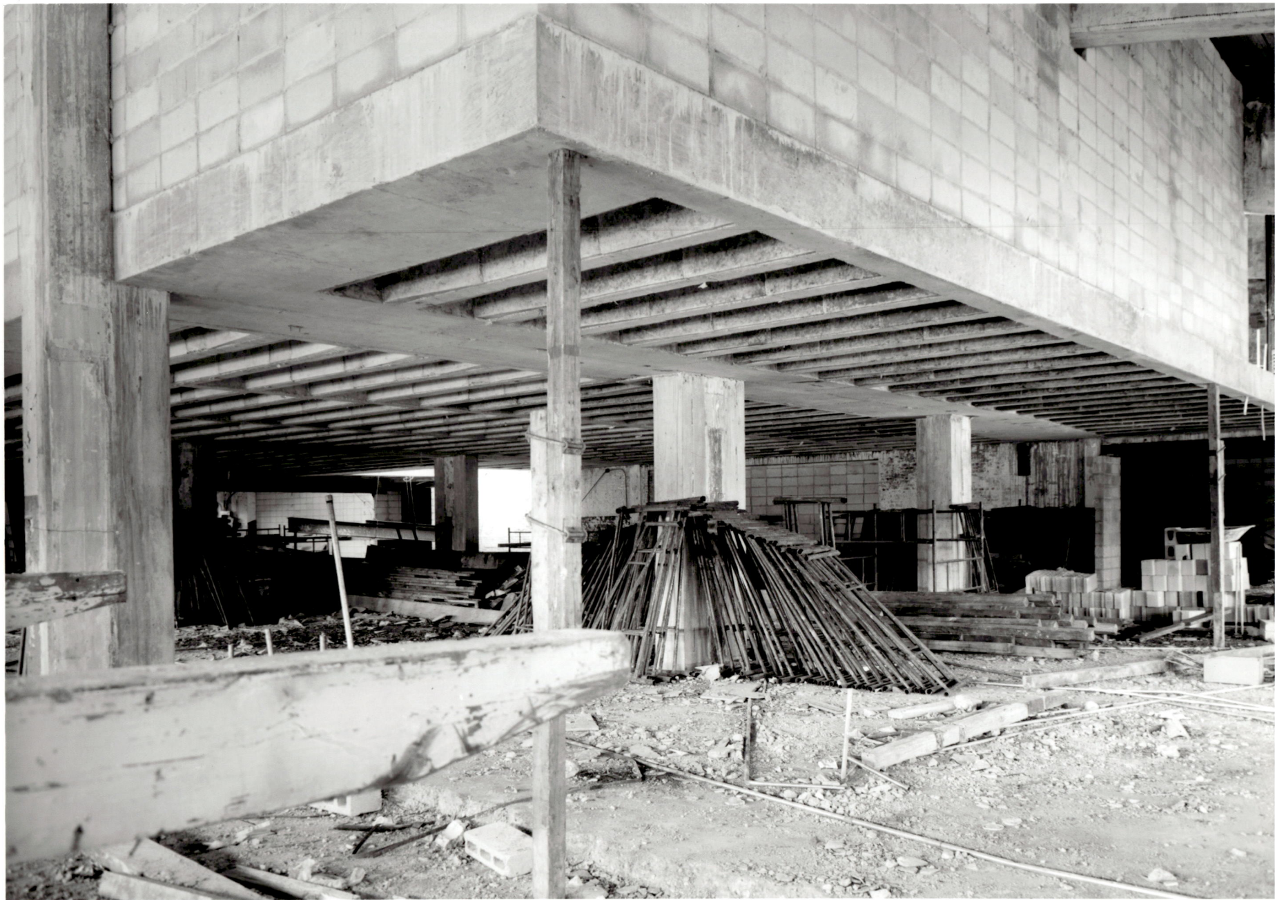
ACADEMIC CENTER UNIVERSITY OF BALTIMORE ROY KIRBY & SONS, INC., CONTRACTOR FISHER, NES, CAMPBELL & PARTNERS, ARCHITECTS MEZZANINE - REMOVAL OF FORMS MARCH 1, 1971
