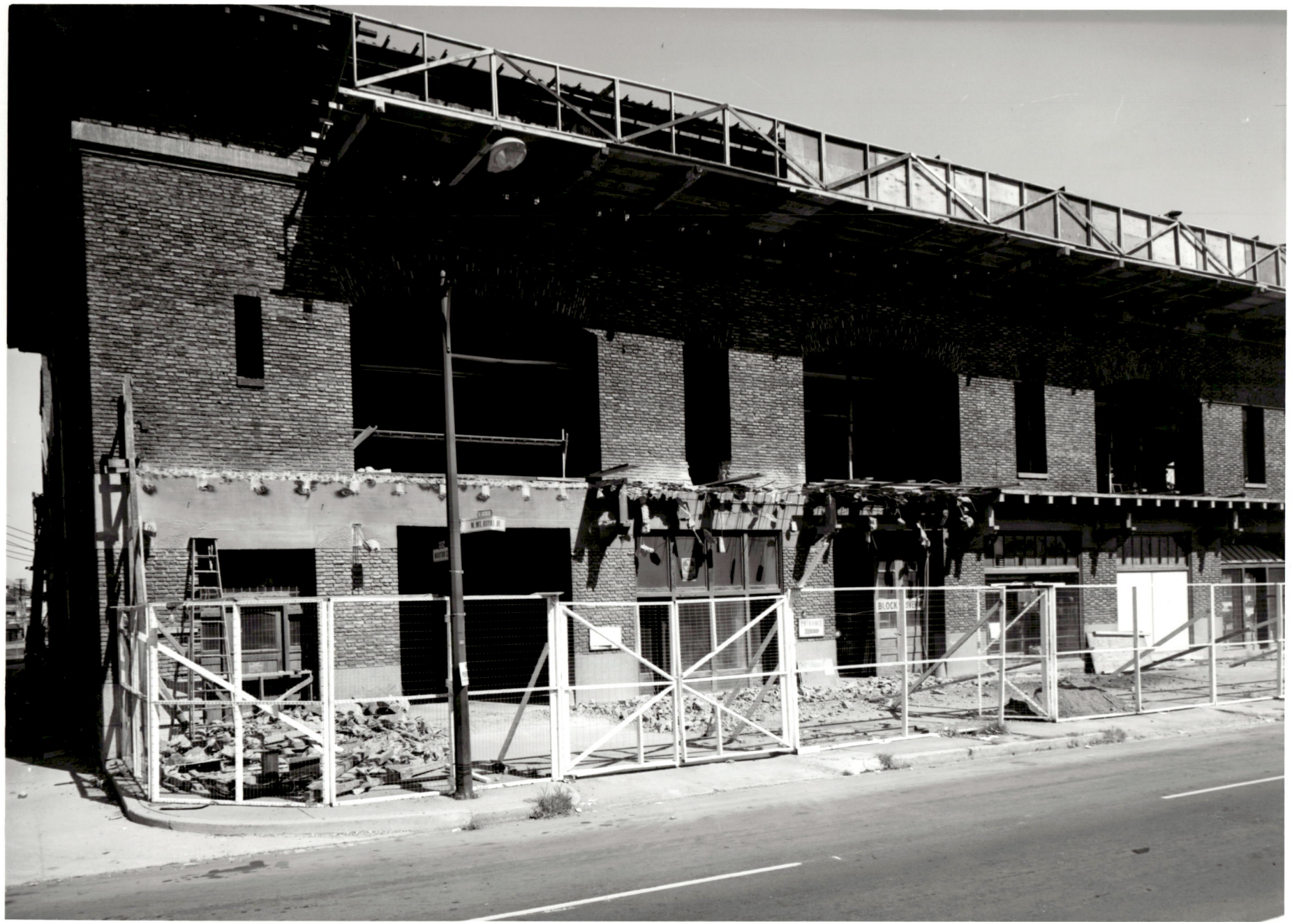
ACADEMIC CENTER UNIVERSITY OF BALTIMORE ROY KIRBY & SONS, INC., CONTRACTOR FISHER, NES, CAMPBELL & PARTNERS, ARCHITECTS REMOVAL SECOND FLOOR BALCONY MT. ROYAL STREET OCTOBER 1, 1970
