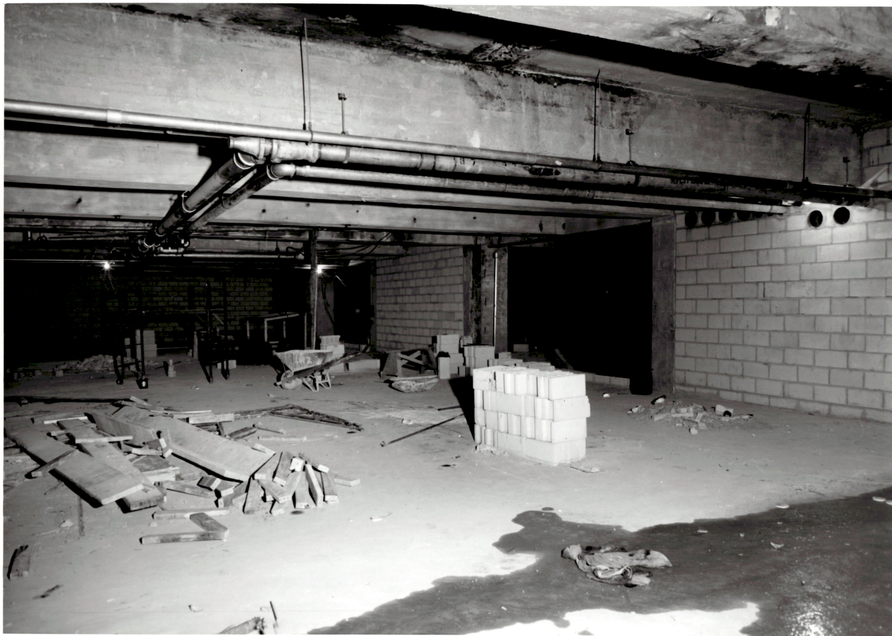
ACADEMIC CENTER UNIVERSITY OF BALTIMORE ROY KIRBY & SONS, INC., CONTRACTOR FISHER, NES, CAMPBELL & PARTNERS, ARCHITECTS BLOCK WALLS GOING UP IN BASEMENT JANUARY 4, 1971
