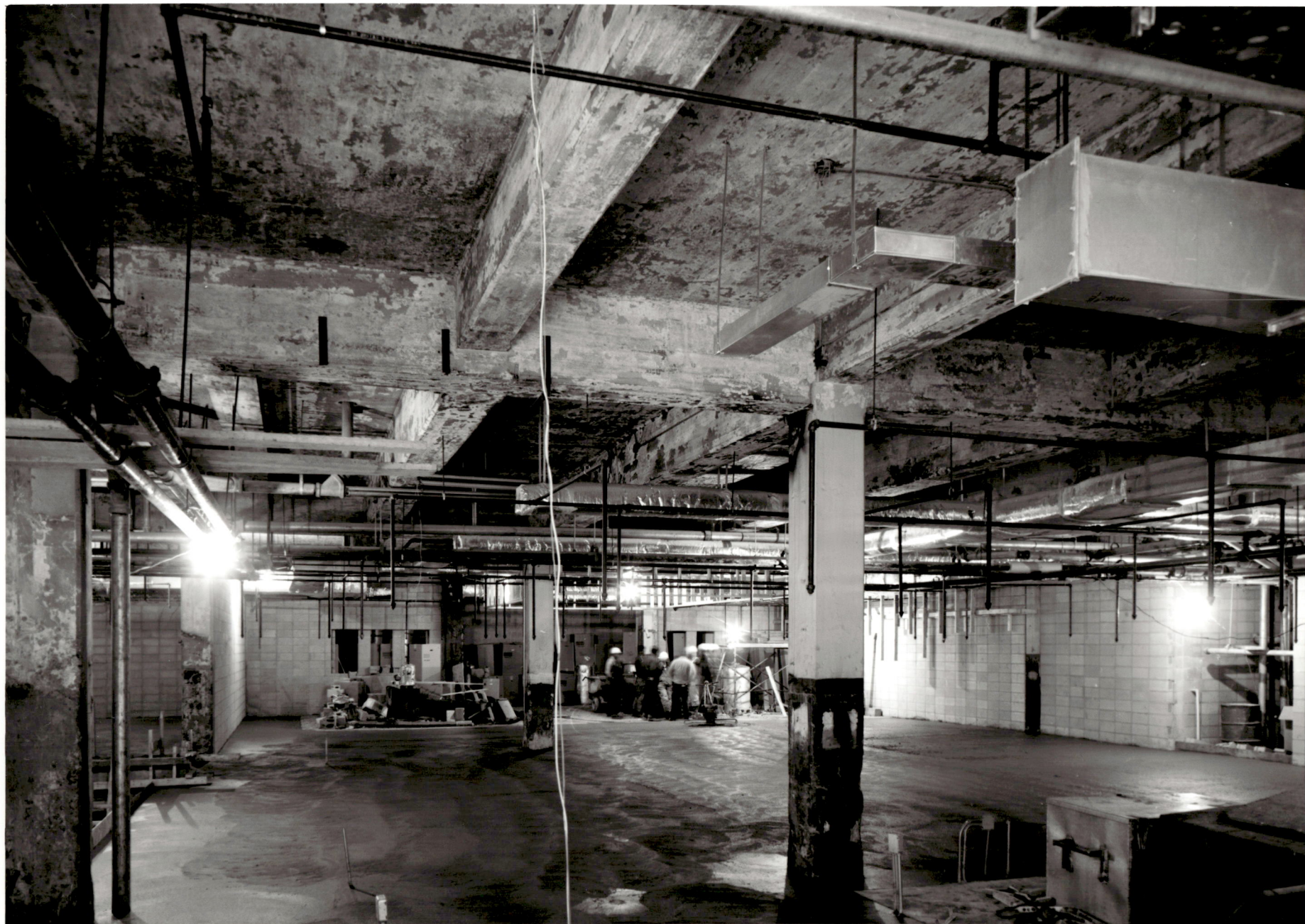
ACADEMIC CENTER UNIVERSITY OF BALTIMORE ROY KIRBY & SONS, INC., CONTRACTOR FISHER, NES, CAMPBELL & PARTNERS, ARCHITECTS NEW FLOOR IN BOOKSTORE MAY 3, 1971
