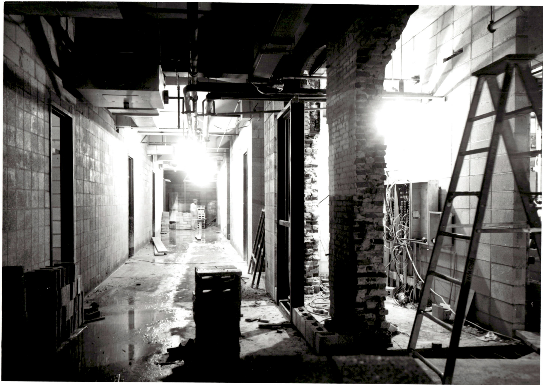
ACADEMIC CENTER UNIVERSITY OF BALTIMORE ROY KIRBY & SONS, INC., CONTRACTOR FISHER, NES, CAMPBELL & PARTNERS, ARCHITECTS SECOND FLOOR HALLWAY AND ELECTRICAL PANELS MARCH 1, 1971
