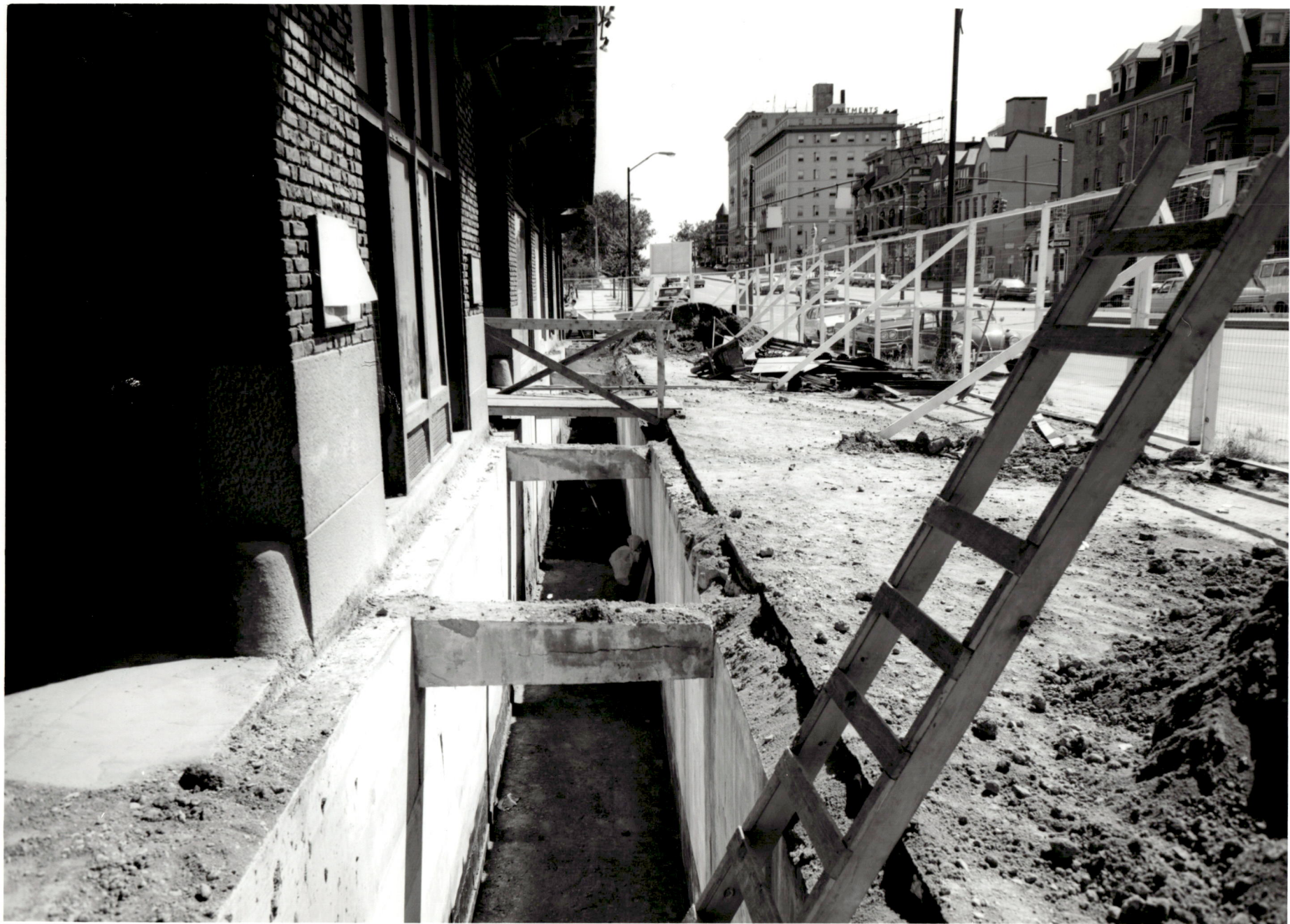
ACADEMIC CENTER UNIVERSITY OF BALTIMORE ROY KIRBY & SONS, INC., CONTRACTOR FISHER, NES, CAMPBELL & PARTNERS, ARCHITECTS THIRD FLOOR DEMOLITION SEPTEMBER 1, 1970
