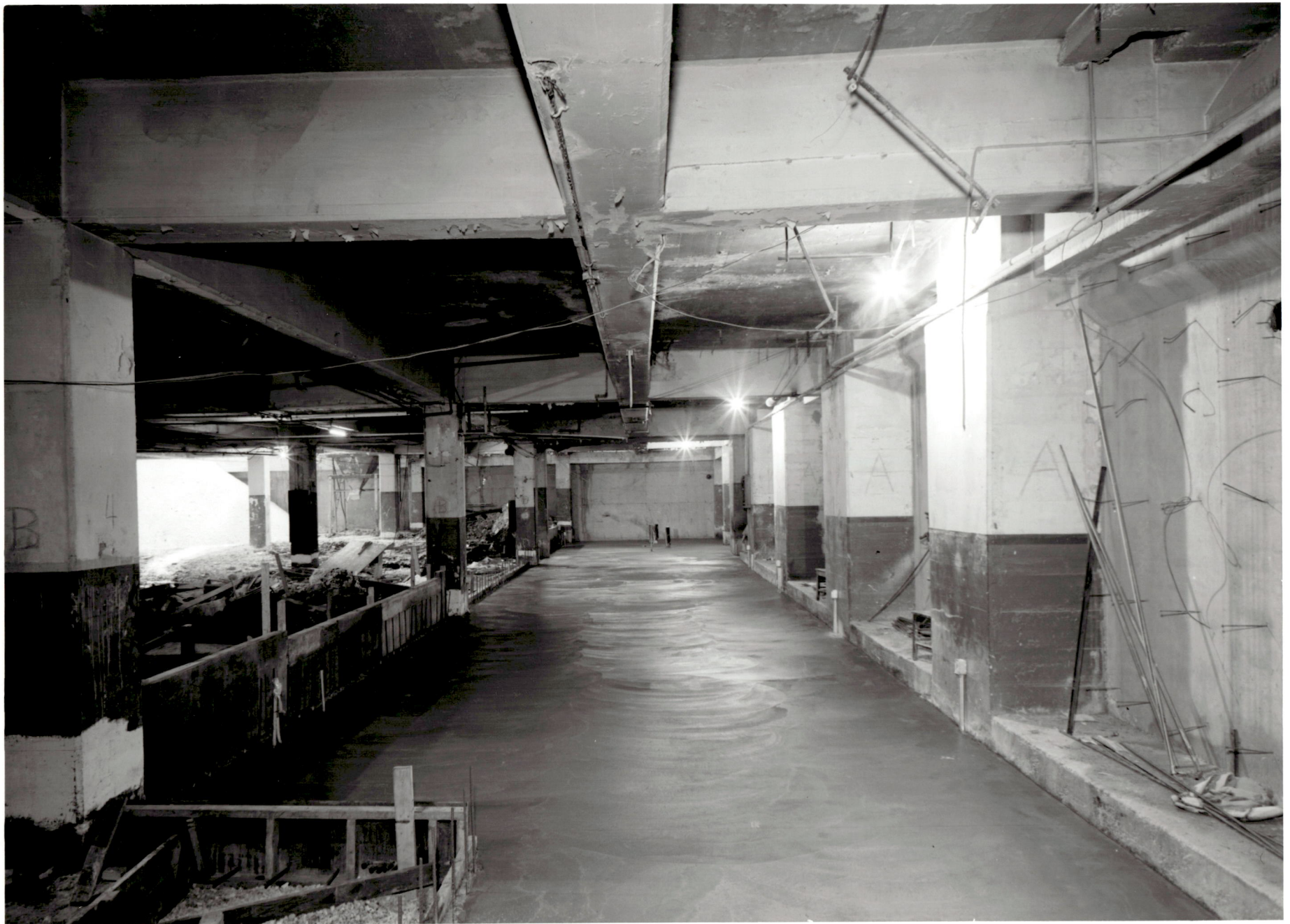
ACADEMIC CENTER UNIVERSITY OF BALTIMORE ROY KIRBY & SONS, INC., CONTRACTOR FISHER, NES, CAMPBELL & PARTNERS, ARCHITECTS NEW SLAB IN TRANSFORMER ROOM NOVEMBER 4, 1970
