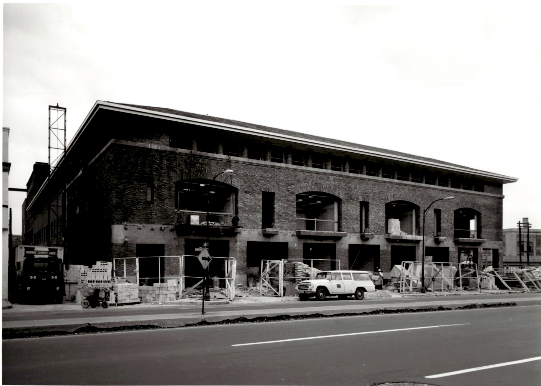
ACADEMIC CENTER UNIVERSITY OF BALTIMORE ROY KIRBY & SONS, INC., CONTRACTOR FISHER, NES, CAMPBELL & PARTNERS, ARCHITECTS GENERAL VIEW LOOKING NORTHEAST MAY 3, 1971
