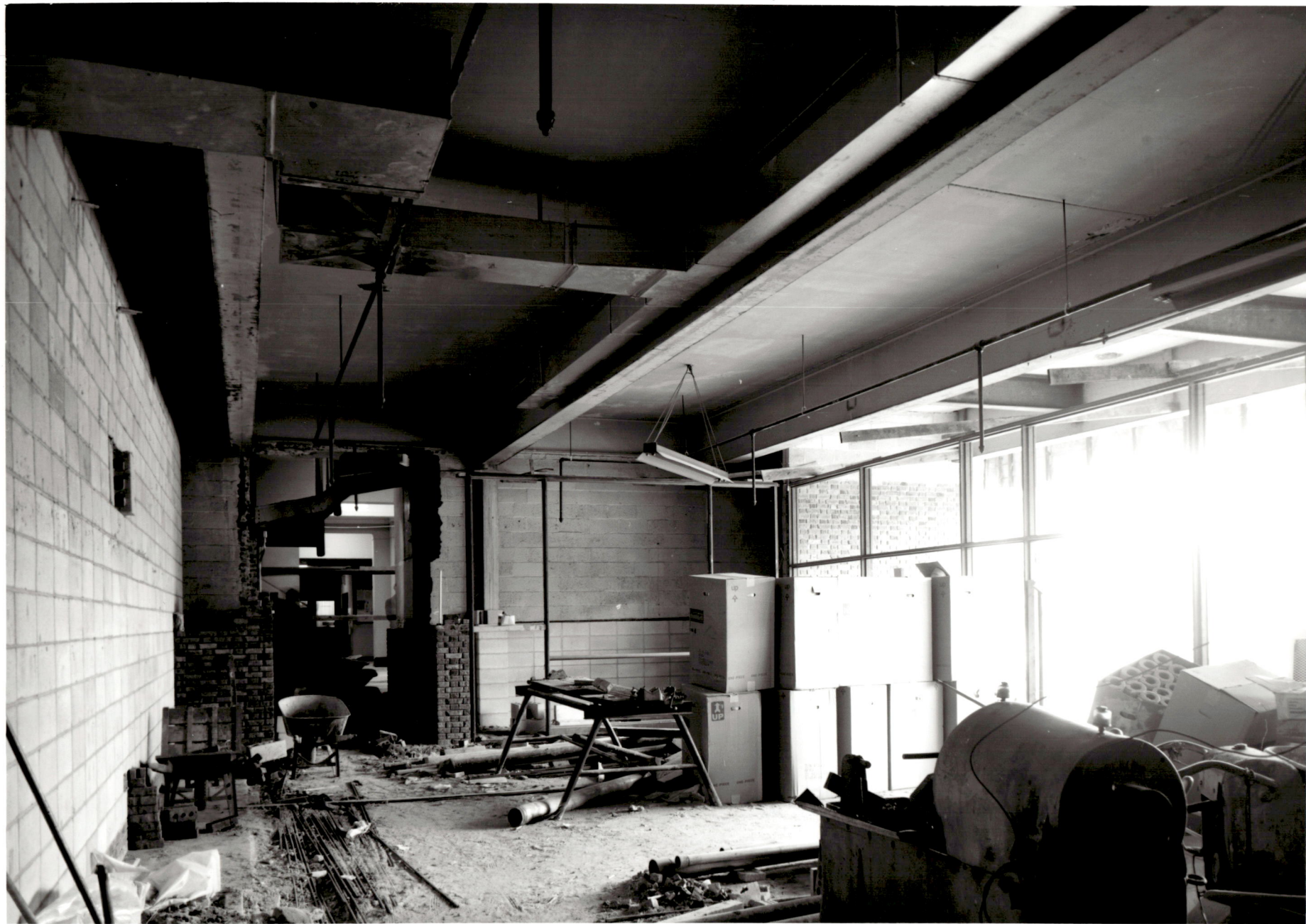
ACADEMIC CENTER UNIVERSITY OF BALTIMORE ROY KIRBY & SONS, INC., CONTRACTOR FISHER, NES, CAMPBELL & PARTNERS, ARCHITECTS GENERAL VIEW OF CHARLES STREET LOBBY MAY 3, 1971
