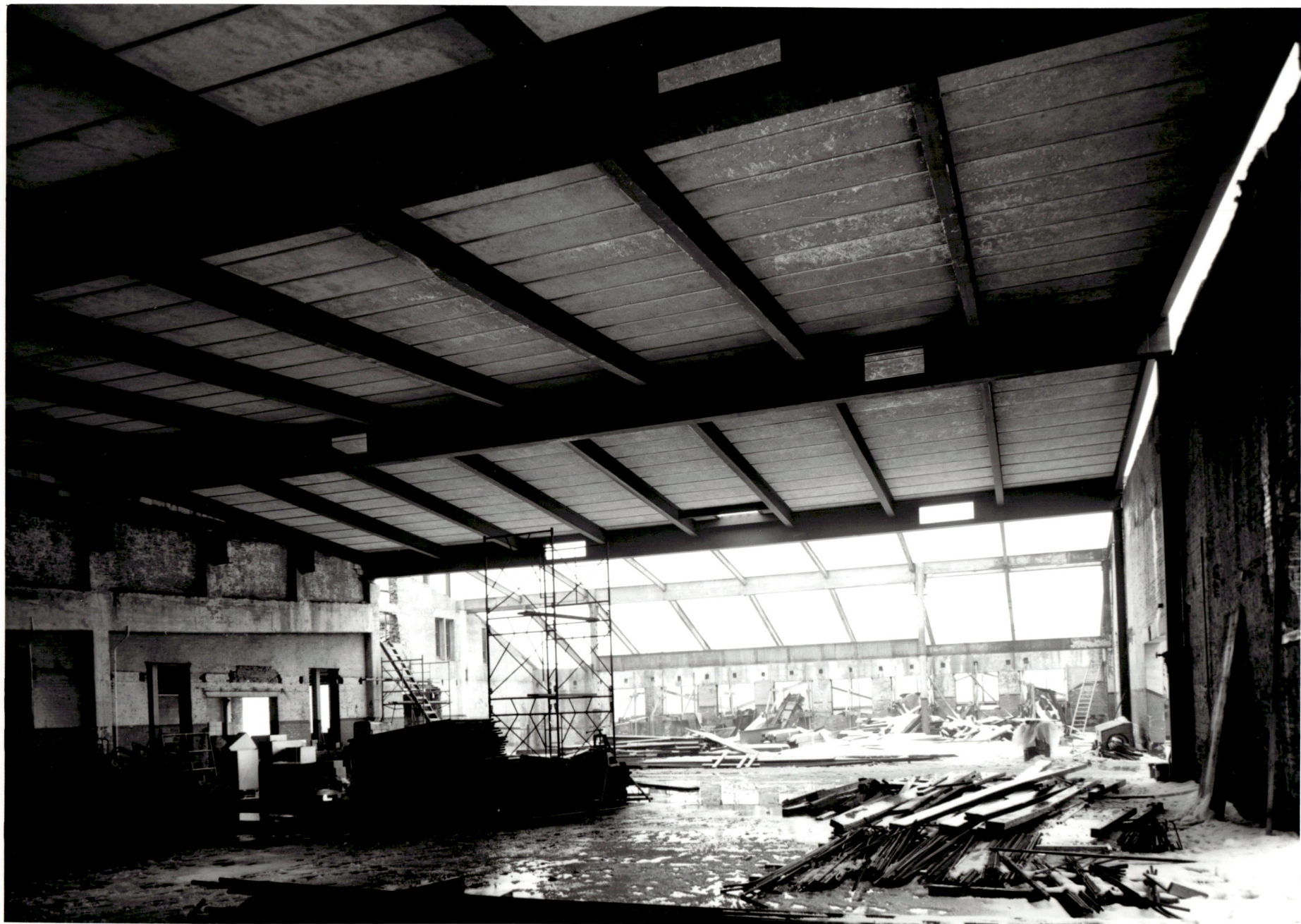
ACADEMIC CENTER UNIVERSITY OF BALTIMORE ROY KIRBY & SONS, INC., CONTRACTOR FISHER, NES, CAMPBELL & PARTNERS, ARCHITECTS NEW ROOF OVER GYMNASIUM JANUARY 4, 1971
