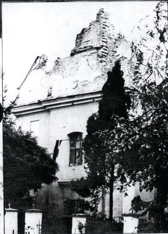
A demolished Orthodox church at Tovarnik... and at Sarvaš.
