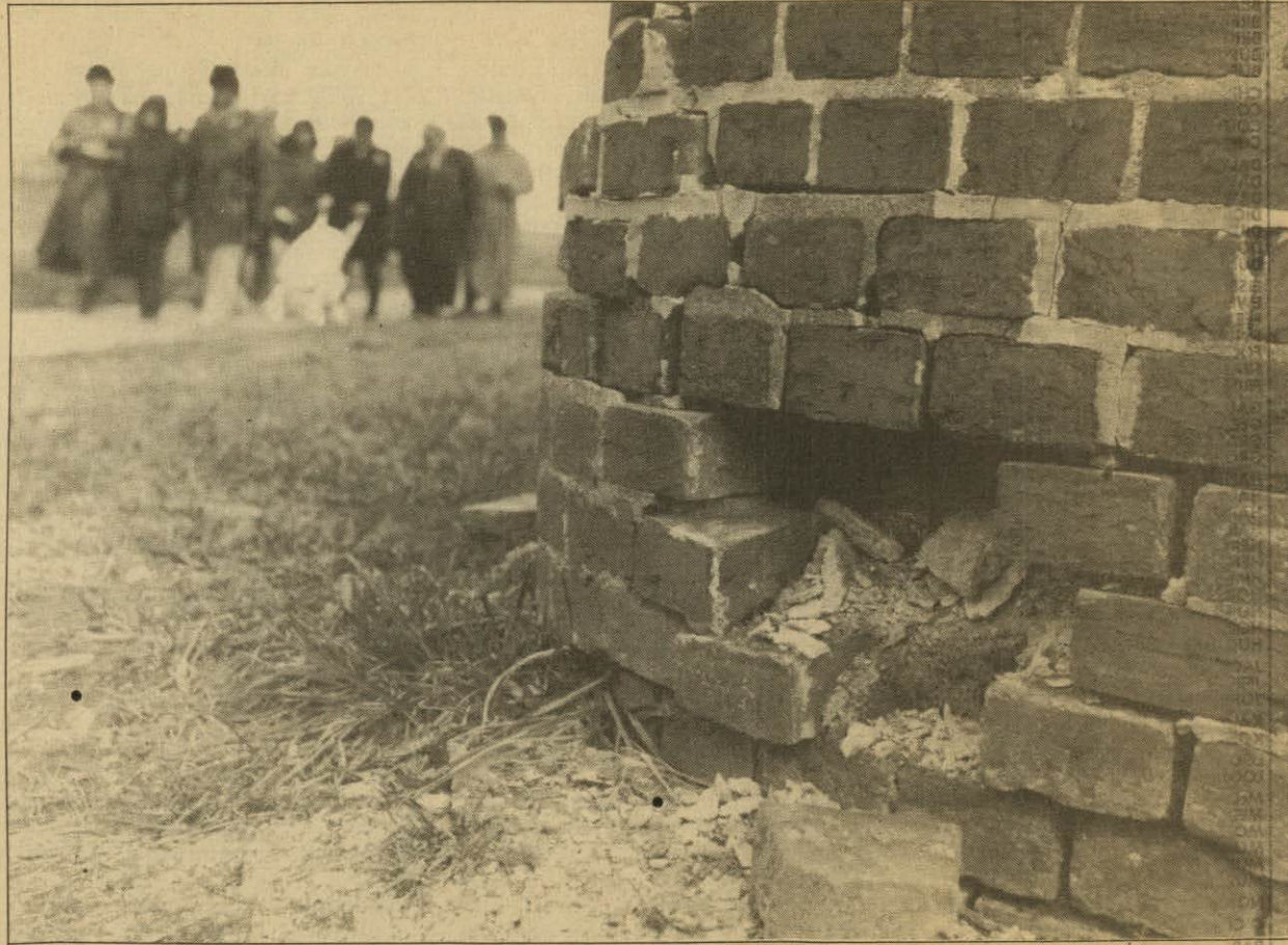
Bricks have fallen from this interior wall at Fort McHenry, which withstood British shells in 1814. The American Legion is raising money for repairs to the monument.
