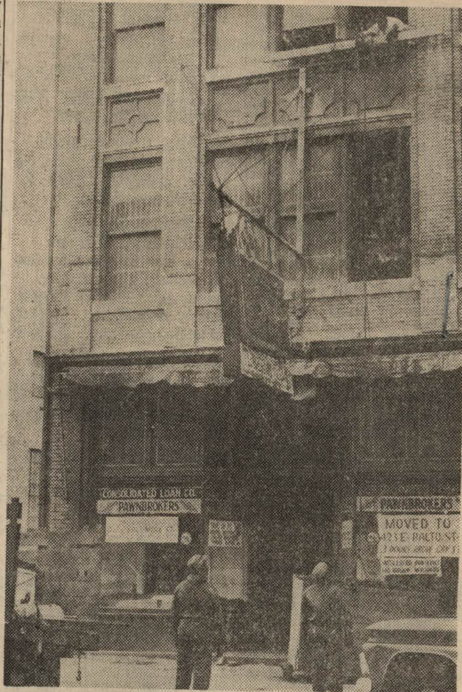
Sunpapers photo—Mortimer MOVED—Workmen move a loan company office from a section of The Block condemned to make way for a redevelopment as a new police headquarters.
