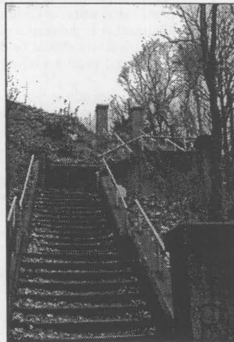
Neglected city steps
